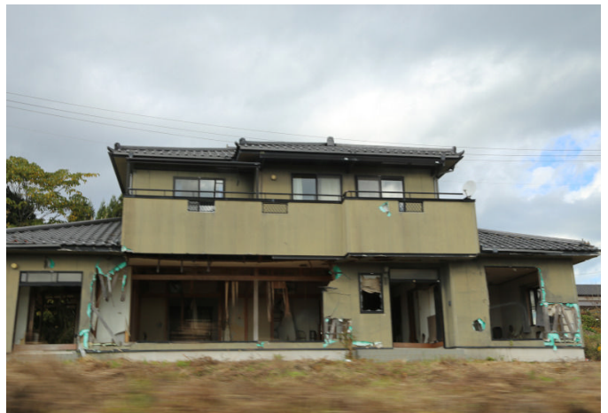
1階は津波で破壊
